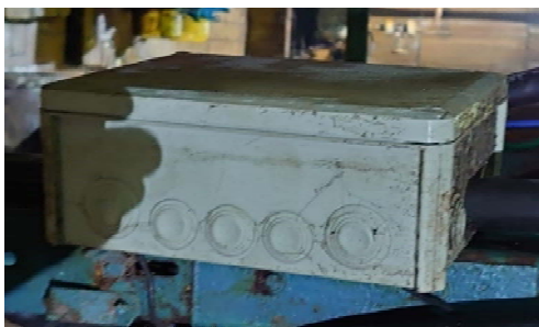
Fig.1 Equipment in normal construction installed in hazardous area classified as zone 2
