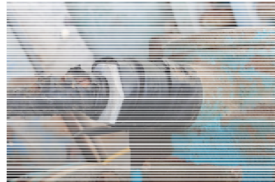
Fig. 4 Damaged cable and cable gland of an Ex d equipment
