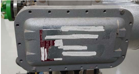
Fig. 3 Bolts missing to an Ex d equipment
