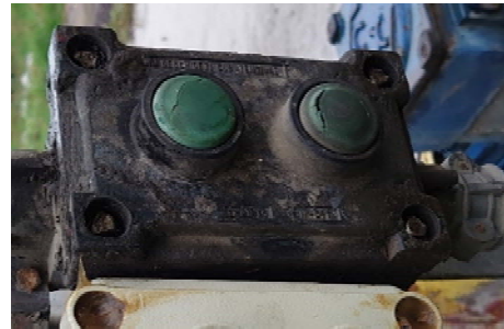
Fig. 6 Damage of rubber elements leading to invalidation of explosion protection for an “Ex de “ equipment
